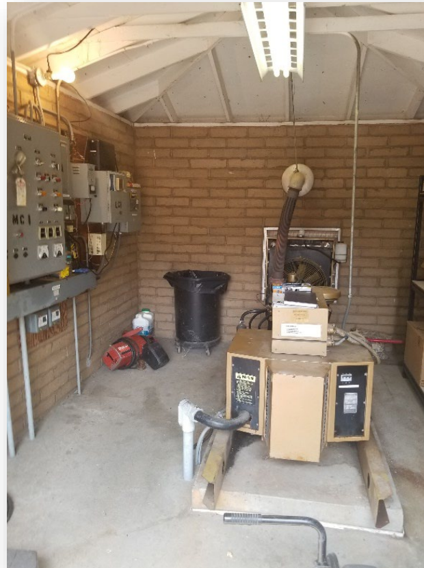
Generator and Building
